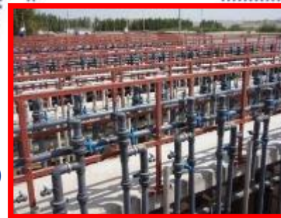
KSA (Sewage, 30,000 m³/d)
