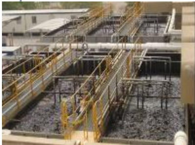
Al Ain, UAE (Sewage, 15,000 m³/d)
